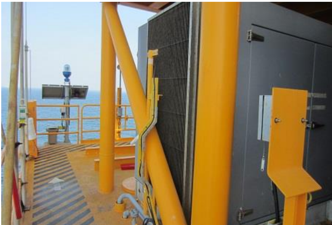
Offshore Unmanned Platform, Class 1 Div. 2 Enclosure. 64kWe Unit in Duabi.
